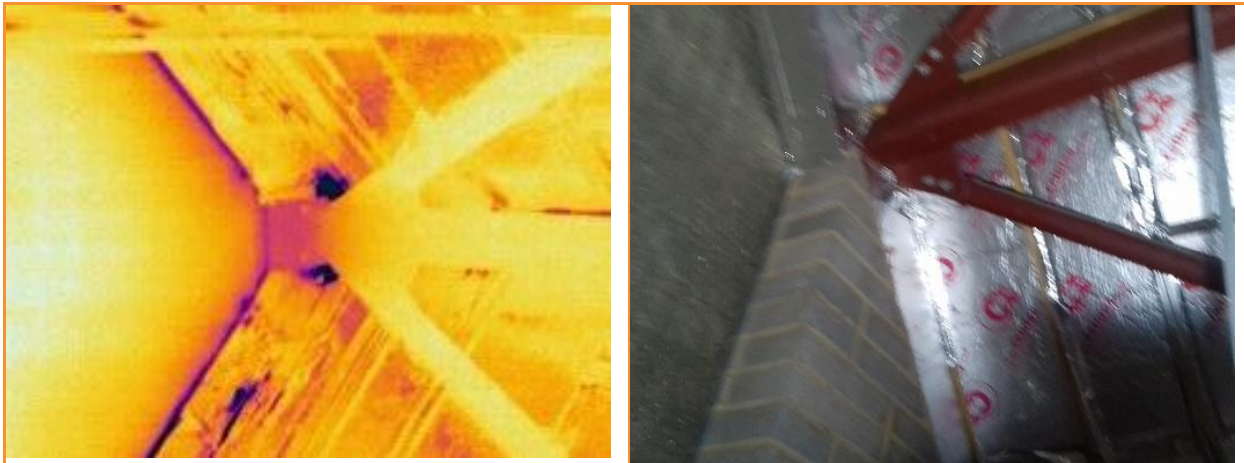
9.26: Thermographic image after pressure applied, of roof space above Sunday School room, cold incoming air clearly visible along top of gable (left side), also above joints in steel frame
