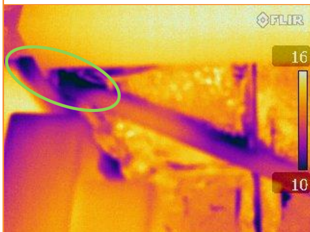
9.34: Thermographic image whilst building depressurised, showing major leak behind joint in steel frame
