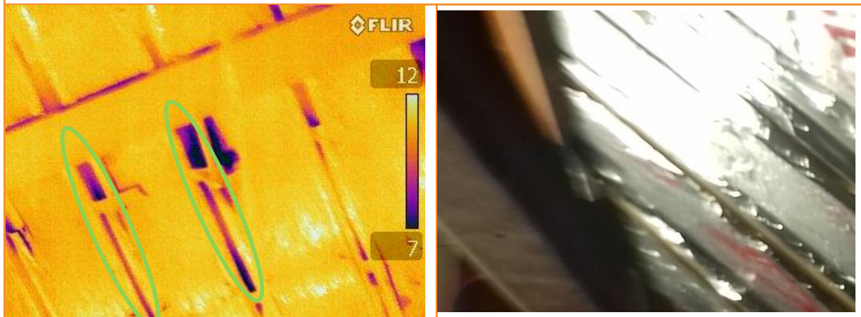
9.37: Thermographic image showing lines of leakage along roof joists where taping has failed, building depressurised
