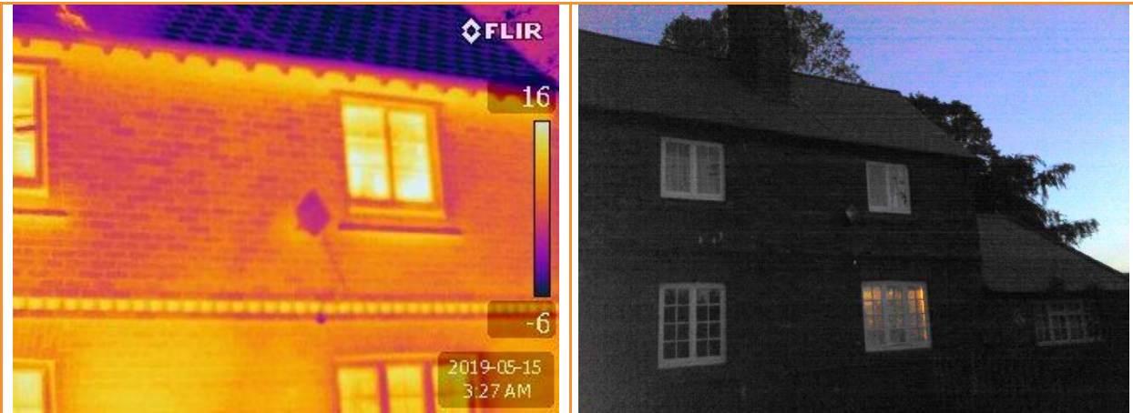
9.06: External thermographic image after house pressurised, showing heat loss along eaves, also along external edge of intermediate floor
