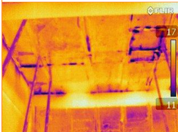
9.40: Thermographic image whilst building depressurised, leakage on many edges of roof insulation pieces where foil taping has failed
