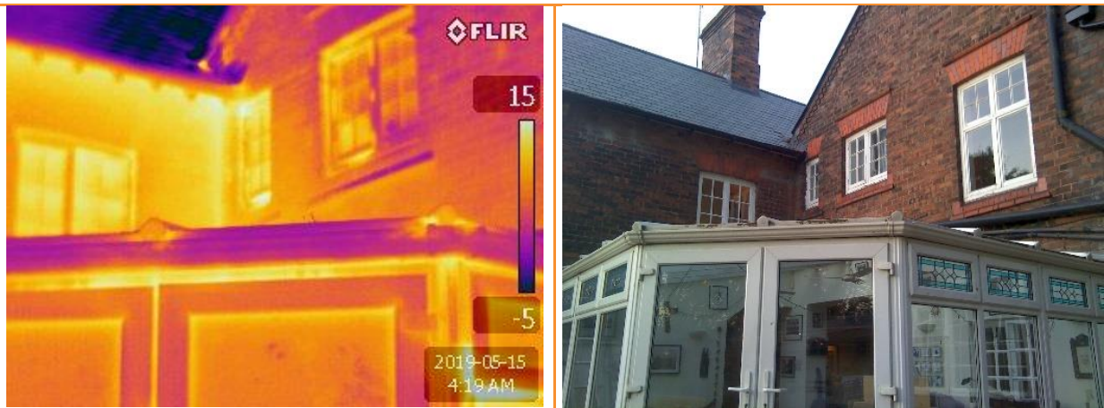
9.04: External thermographic image after house pressurised, showing increased heat loss along eaves, also around top of conservatory and at ends of conservatory roof structure
