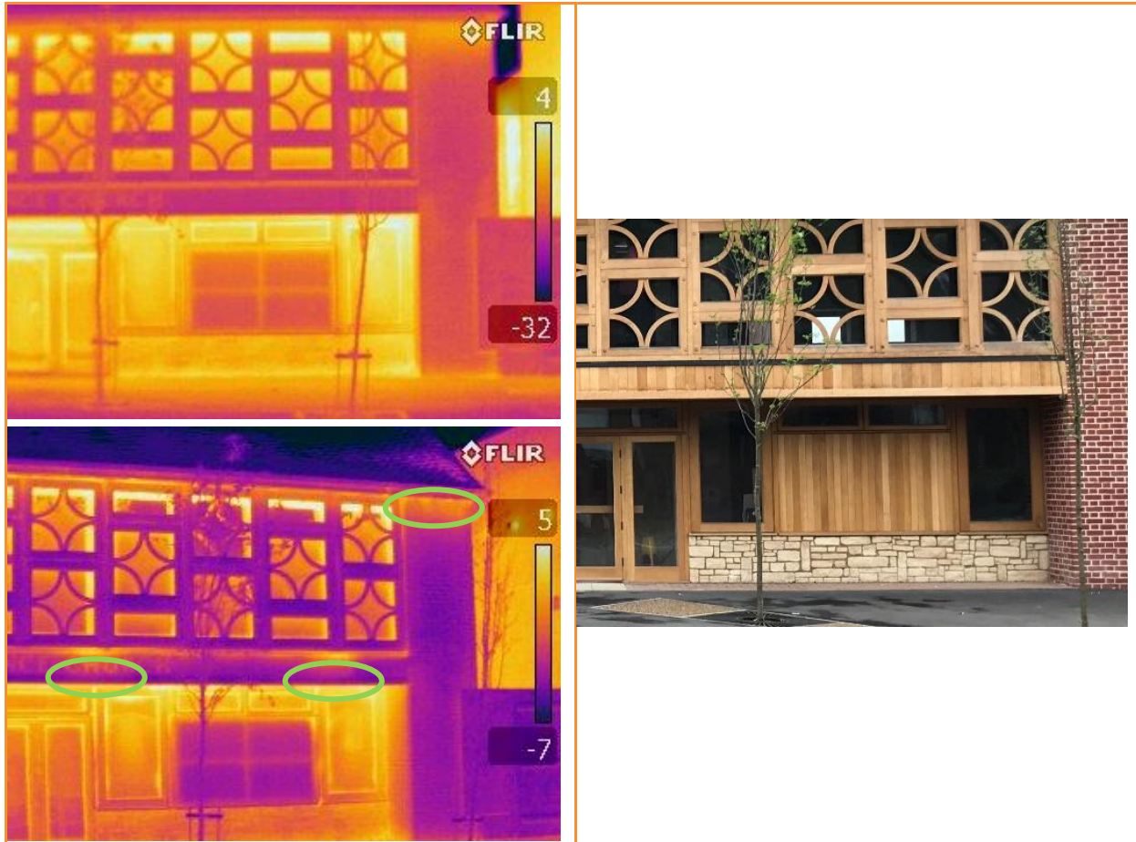
9.16: Leakage along underside of balcony and along eaves visible behind upper window frames, before building pressurised (top), then after building pressurised, showing more leakage along underside of balcony, and at top of brick column at right hand side (bottom)
