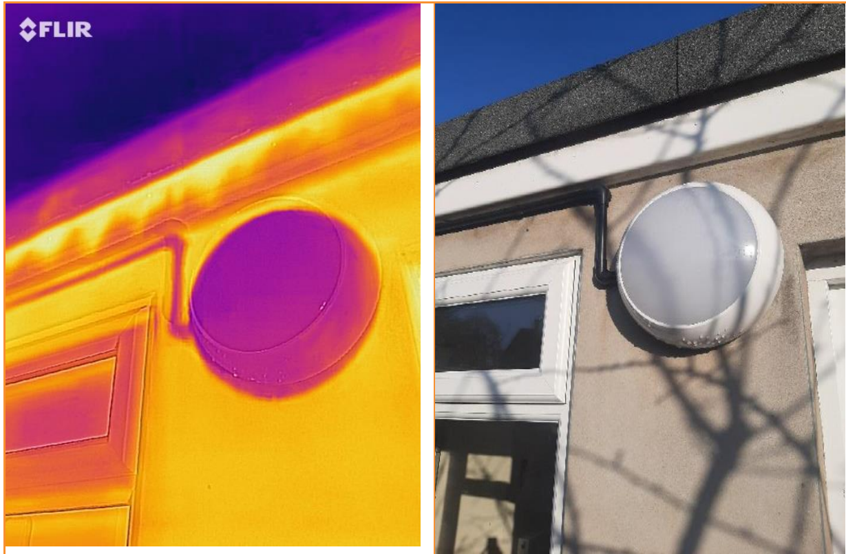
9.08: External thermographic image whilst building pressurised, showing considerable warm air (white/yellow) escaping along the bottom edge of eaves to the rear flat roof extension
